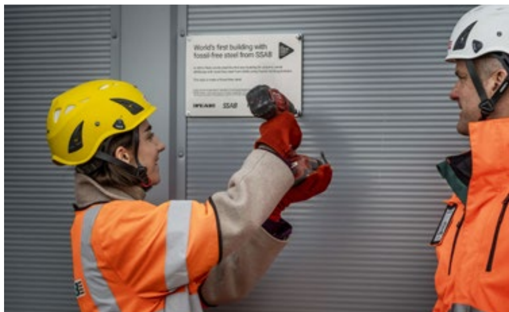
Sweden's Minister for Climate and the Environment, is screwing on the sign for the project together with Peab's Business Area Manager Construction, Stefan Danielsson. The project was commissioned by real estate company Wihlborgs and the building will be ready to move into in the spring of 2024.
