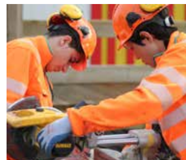
There are around 430 students annually in the construction and civil engineering program at the five Peab Schools located in Ängelholm, Malmö, Gothenburg, Solna and Upplands Väsby.
